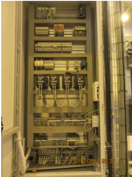
Figure 35 The electric cabinet
